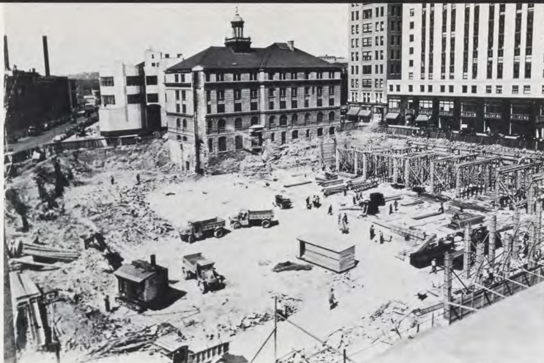
Construction is underway in this 1931 photograph which also shows the recently-razed county jail.
