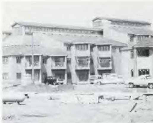
Atrium condominiums under construction in 1983. Lanterns along the roof ridges repeat lanterns used to light interiors of shops.
