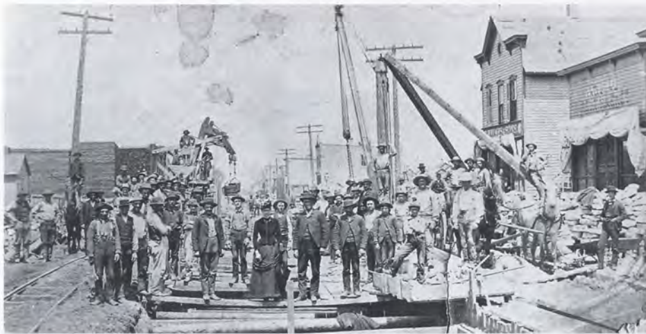
Laying a sewer in Rice Street ca. 1880 — another beneficiary of Flanagan's tax payments.
