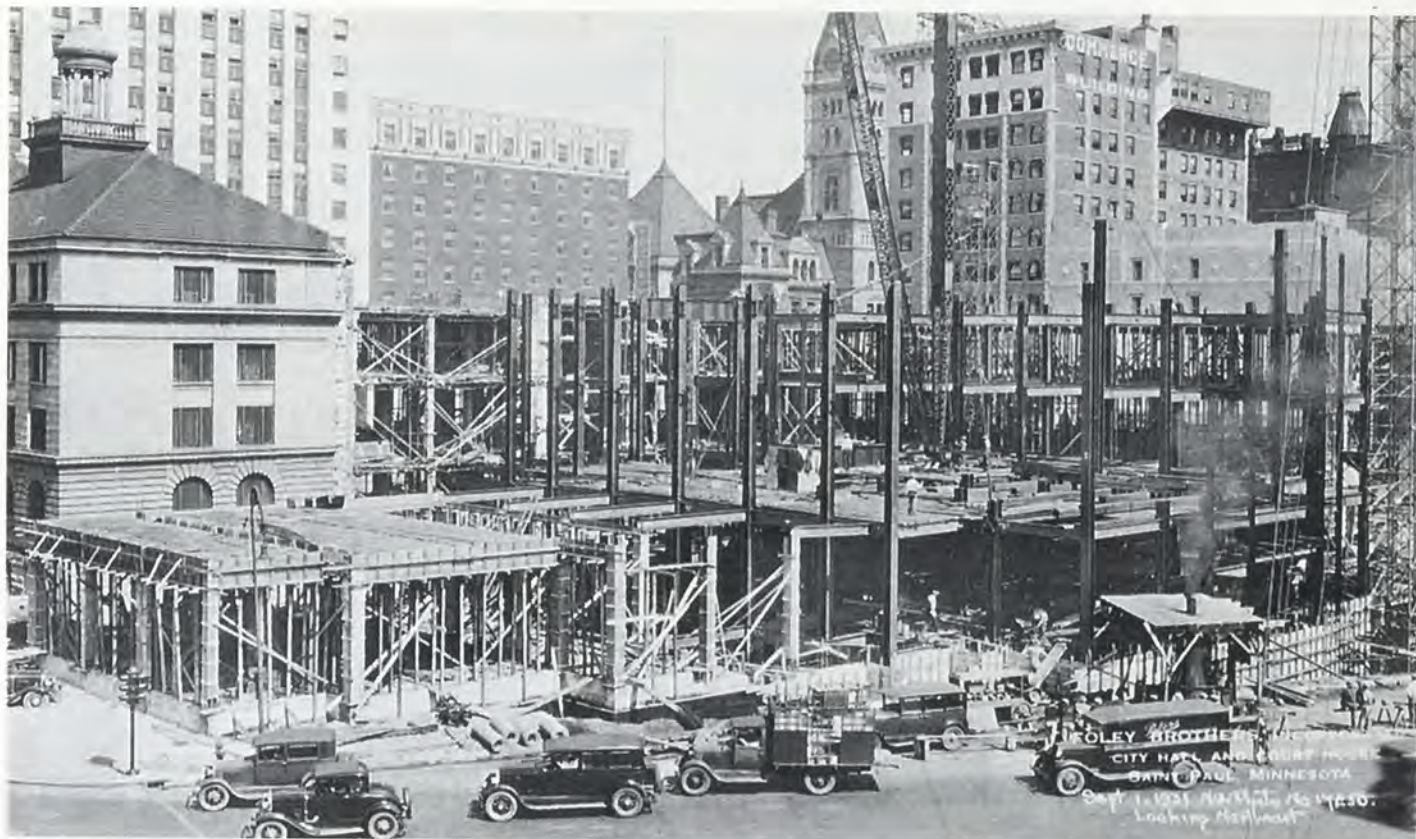
St. Paul's new City Hall/County Courthouse goes up in 1931. Will Oppenheimer was a leader in the drive to build the new courthouse. Minnesota Historical Society photo.
