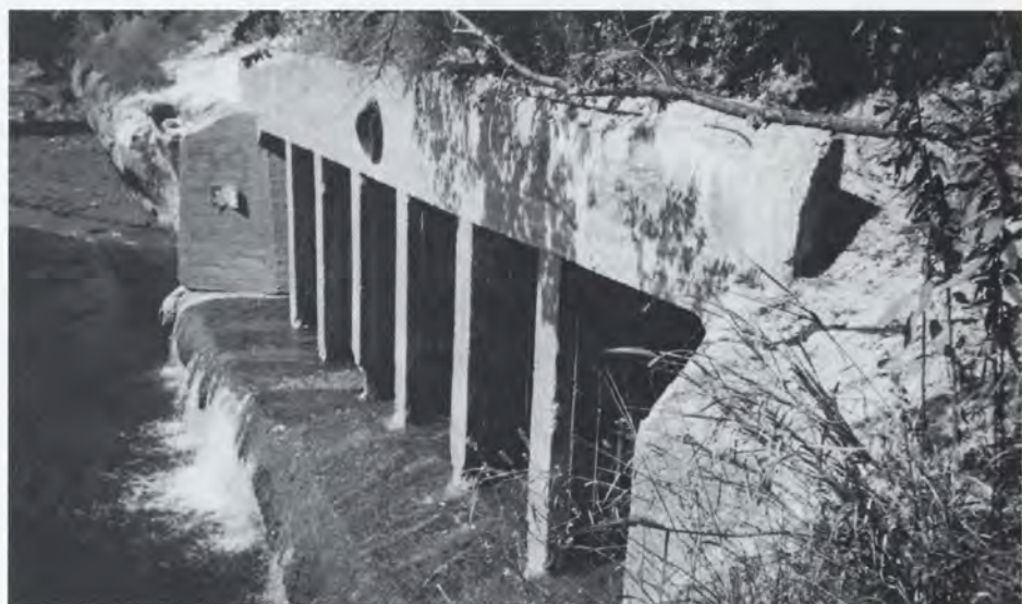
The Bay Street outfall. While other streams in St. Paul have been put underground, none has undergone such drastic reroutings as Cascade Creek, which currently joins the Mississippi three-quarters-of-a-mile upstream from its original junction with the river. Photo by the author.
