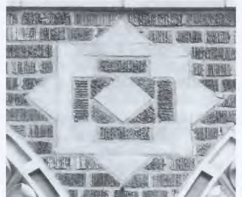
Detail, between windows, front of building, St. Anthony Park Free Public Library, 1917. Photo courtesy of Lauren M. Freese.
