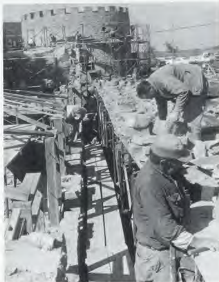
Restoration and rebuilding of old Fort Snelling underway in October, 1966. Photograph by Alan Ominsky, Minnesota Historical Society.
