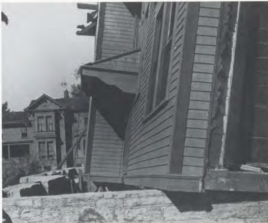
Off its Base. The tornado that roared through St. Paul on August 20, 1904, lifted the old T. B. Campbell residence from its foundation at Woodward and Monroe Place. According to news accounts, three occupants were inside at the time. Minnesota Historical Society photo.
