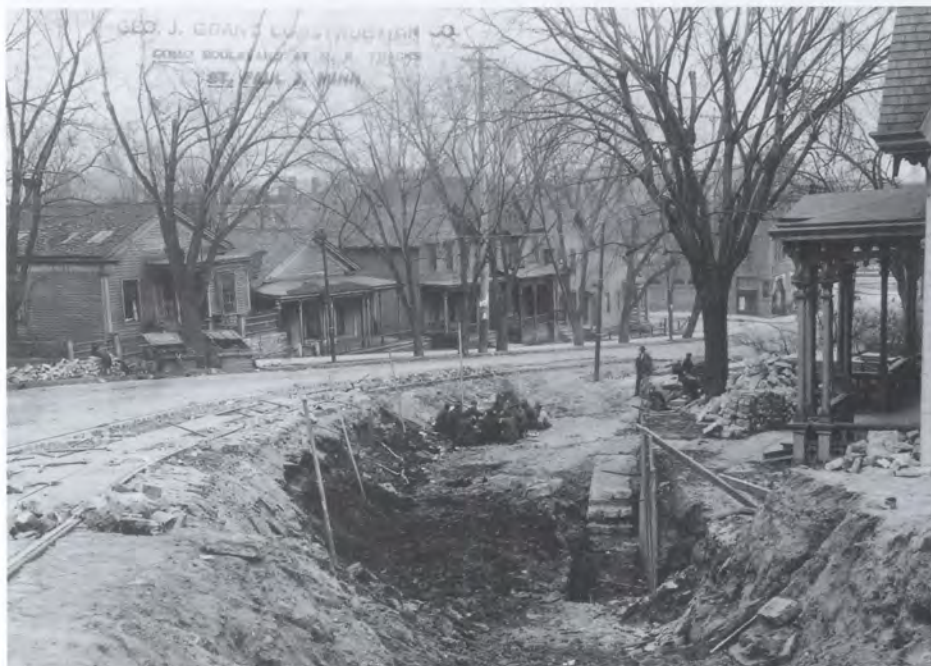
Another view of the construction of the tunnel's lower entrance looks toward the southeast at the junction of Selby and Third Street. Simple frame houses line Third Street across from the Gilman residence.
