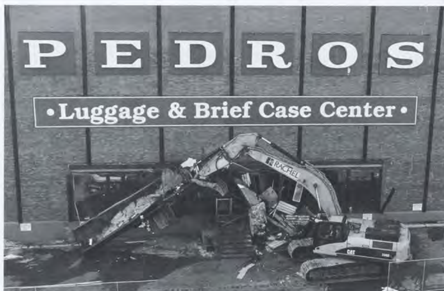
This photo from 2011 shows the start to the demolition of the Pedro Luggage store. Eventually this site will become Pedro Park in downtown St. Paul. Photo courtesy of Minnesota Public Radio.
