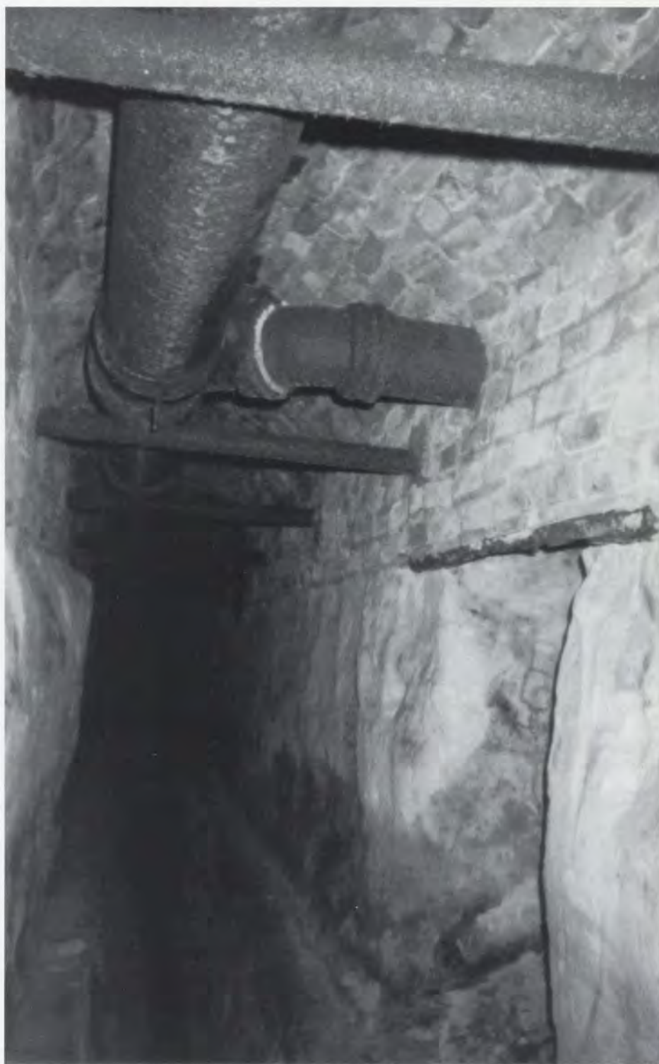
The Omaha sewer tunnel today. This photo by the author shows the Fountain Cave plumbing system. Strother's pipe runs along the ceiling. This sandrock tunnel was given a brick arch at places where it grazed the overlying tumblerock layer. The opening along the right wall leads to a sinkhole under the former Machine Shop. Initially, cavers thought that "sinkhole K" (point K on Strother's map) would provide a backdoor into Fountain Cave.
