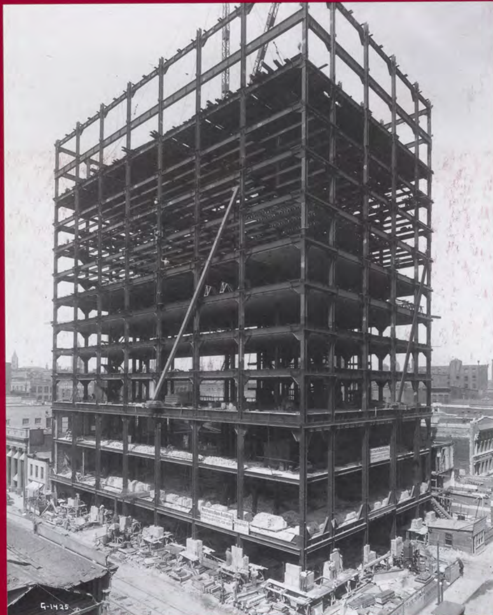
The Merchants Bank building under construction at 333 North Robert Street in 1914. Photo from the Minnesota Historical Society. See article beginning on page 4.
