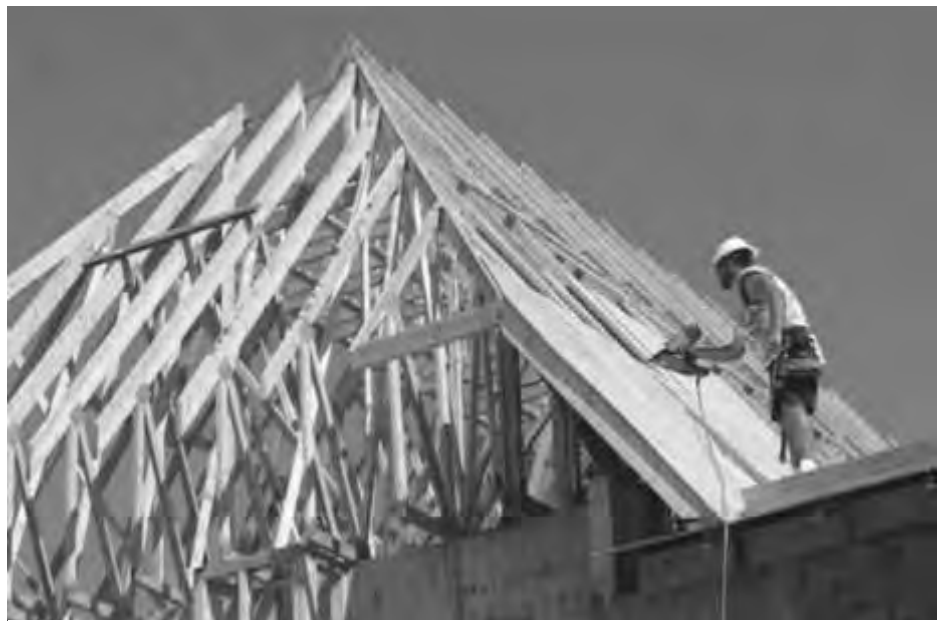
A recent photo shows a roofer using an air-powered nailer attaching plywood sheets to building trusses manufactured by Villaume. The small silver sheets mounted on various truss joints on the left are the famous "Gizmo Gussets," or metal connector plates, that helped make custom-designed trusses practical, effective, and affordable.
