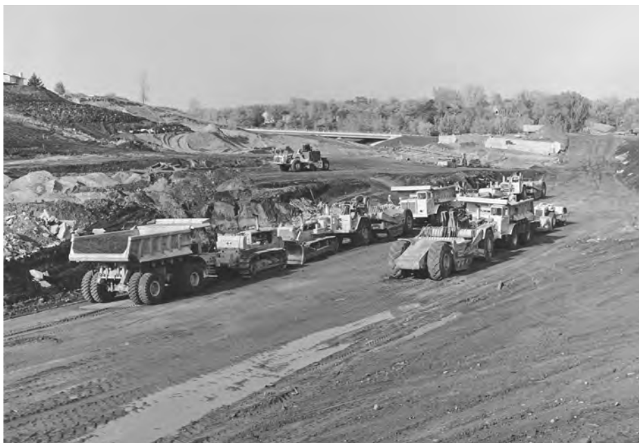
By 1971 construction of I-35E had moved northward across the Mississippi. The Randolph Avenue Bridge over the route for the new highway can be seen in the background. Bridge construction typically preceded construction of the roadbed. Henry B. Hall photograph. Photo courtesy of the Minnesota Historical Society.
