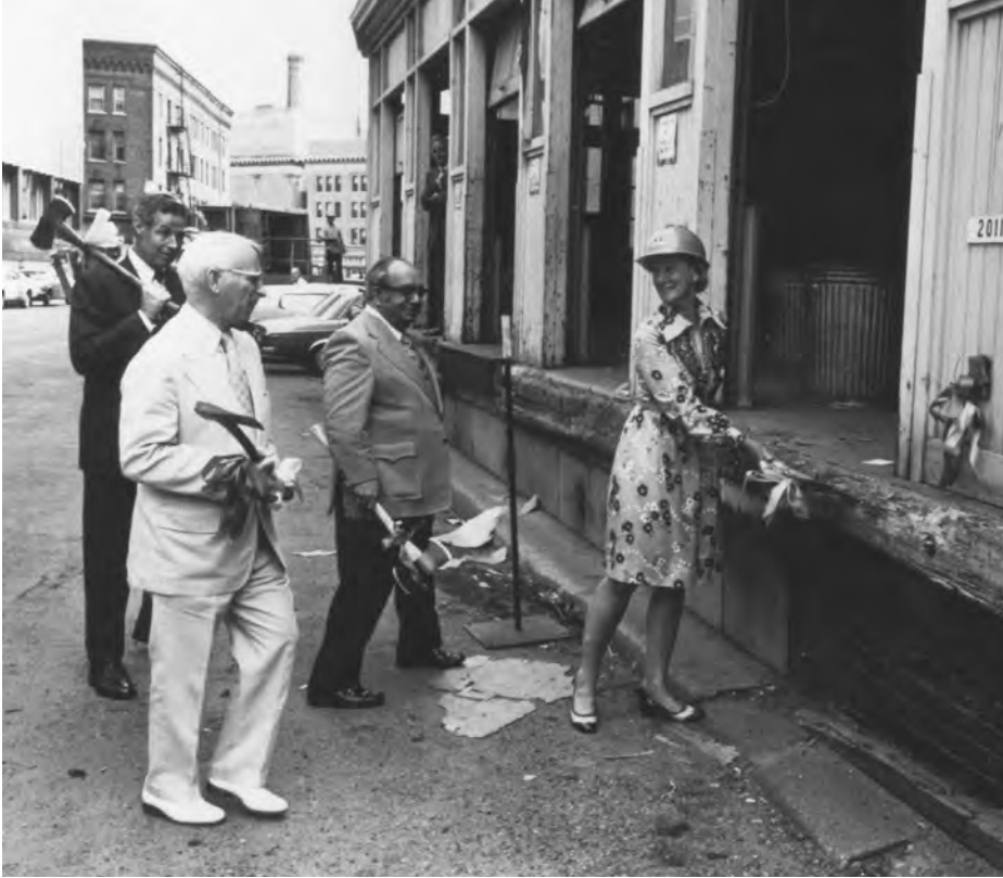
The restoration of the Old Federal Courts Building on Rice Park in downtown St. Paul was a massive project. In this photo from 1975, the hard work of making the building into Landmark Center began with Elizabeth Musser, right, the chief fundraiser for the nonprofit that would operate the building, striking the first ceremonial blow on what was then the loading dock of the former post office, which faced Washington Street. Ready to follow her example are, left to right, Carl Drake and Ron Hubbs, both of the St. Paul Companies (now Travelers) and Frank Marzitelli of the St. Paul Port Authority. Photo by Joan Larson King. Photo courtesy of Minnesota Landmarks.
