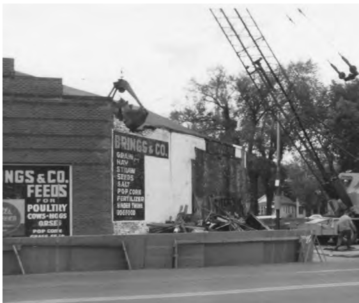
Demolition of the Brings and Company building began on February 1, 1971. Truly a sad ending to a popular St. Paul company that spanned 114 years and four generations. Today the Sherman-Forbes Housing occupies this site. Photo courtesy of the Kremer Family Collection.
