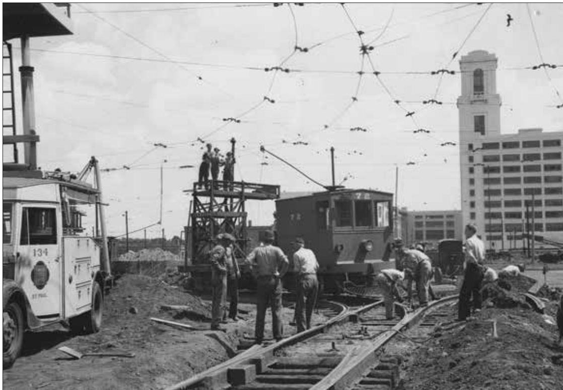
Looking east, workers relocate tracks and overhead trolley wires in the Snelling storage yard in the summer of 1949. Traffic congestion forced abandonment of the entrance at Snelling and University Avenues and the construction of a new entrance on University east of Snelling. Wire car 72 was built at the Snelling Shops. It and all TCRT work equipment will be scrapped when the shops close six years later. Prior to the construction of Allianz Field, a restaurant stood near this location for many years. Photo courtesy of the Minnesota Historical Society.
