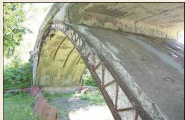
This image illustrates the Melan system. A three-span, open-spandrel, reinforced-concrete, barrel-arch bridge, its reinforcement consists of five latticed Melan ribs in the arch ring with Thatcher bars in the piers and floor slab. Courtesy of Dr. Robert Frame, Mead & Hunt.
